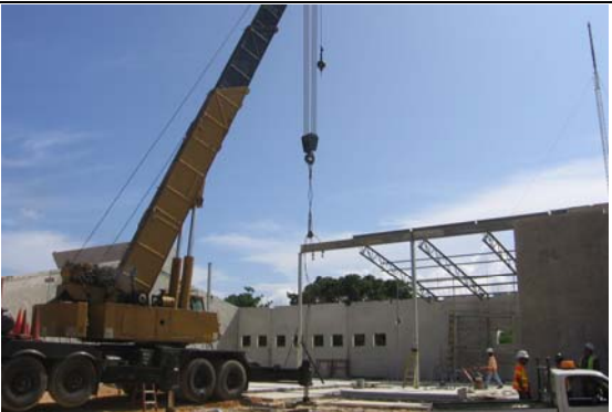
2A: Sheet metal roofing deck material staging area. 2B: Crane positioned to install internal pre-cast walls.
